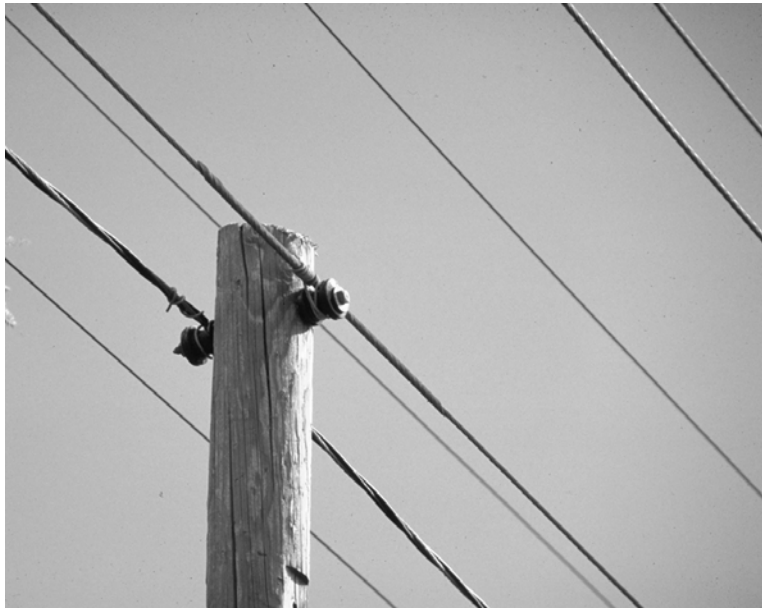
Figure H234B Skip-span pole not having vertical clearance required by Rule 234B2 of horizontal clearance at the structure required by Rule 235B
