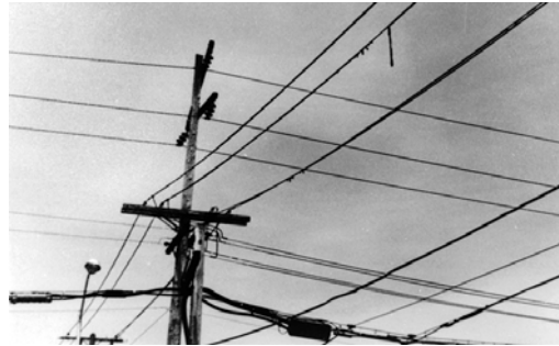
Figure H230-7 Covered conductor with deteriorated covering
